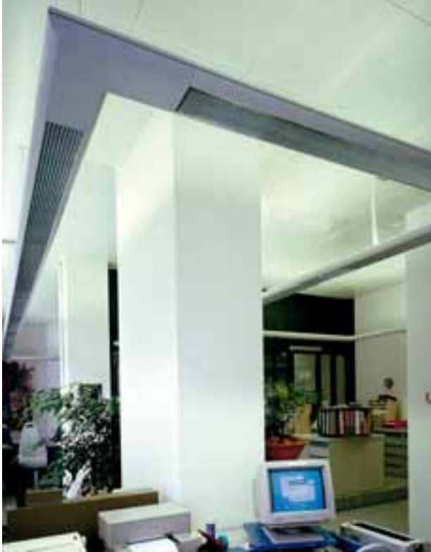
Glare free lighting created by parabolic louver P 13
